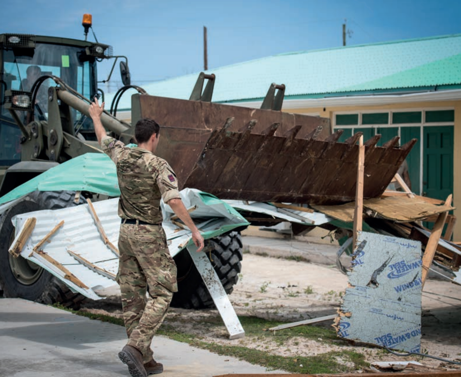
Pictured is E.L. Simons Primary School being cleaned up ready to be repaired after the damage caused by hurricane Irma. RFA Mounts Bay offered support to Grand Turk island in the Turks and Caicos islands, in support of the Commando force from 3 Cdo Brigade personnel from 40 Commando Royal Marines and 59 Commando Royal Engineers. Photo: Corporal Darren Legg, Crown Copyright.
